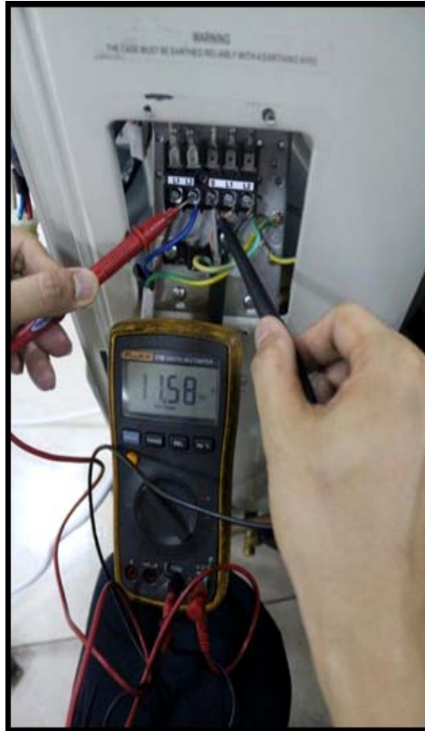
Fig. 32 – Test the DC Voltage
